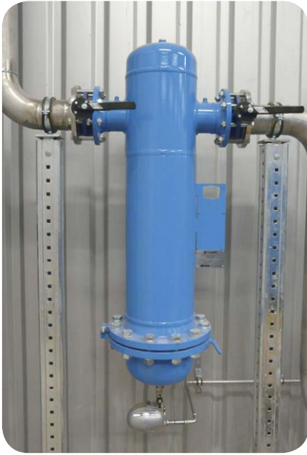
Refrigerant dryers and filters support centralised preparation of oil-free compressed air.
